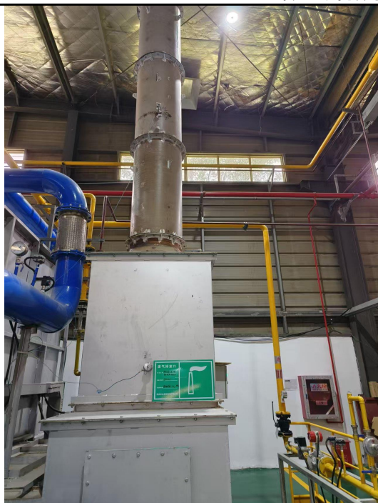
废气排放口标识牌-高温煅烧DA001
