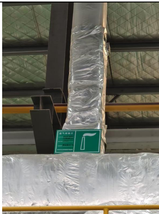
废气排放口标识牌-烘干DA006
